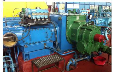
New crankcase and cross head guide in operation
