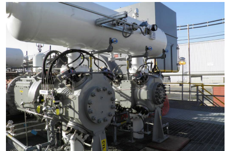
HydroCOM actuators on the compressor
