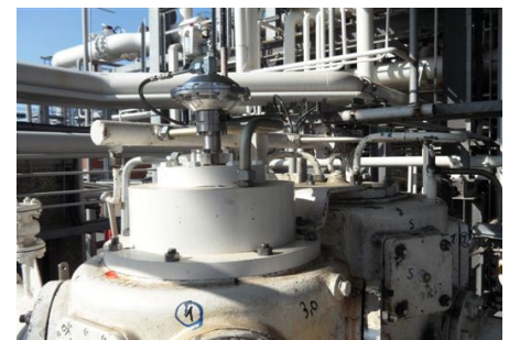
New control system in place on the cylinder
