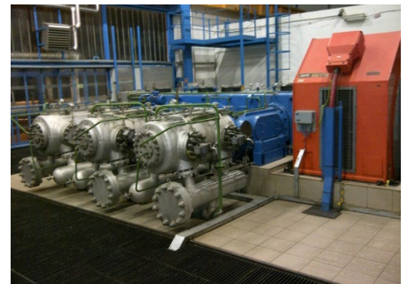
6-crank machine with HydroCOM and monitoring system
