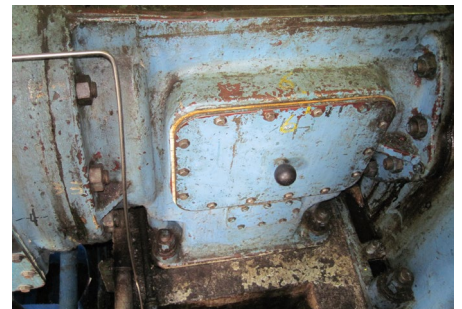
Old, cracked crosshead guide
