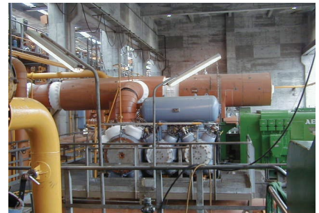
One of the two propylene compressors
