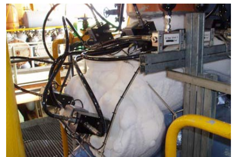
Actuators covered in ice during operation
