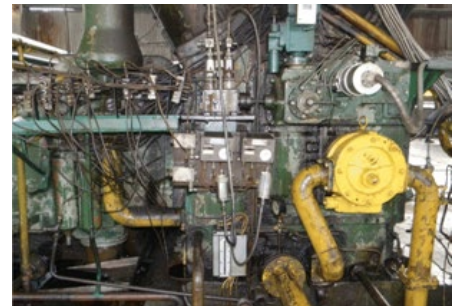
Old lubrication system
