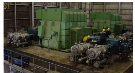
Overhauled compressor with low bearing temperatures
