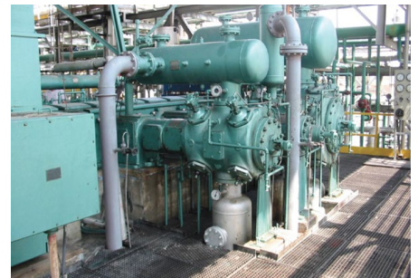
Booster and primary compressors
