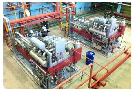
Both compressors running on site
