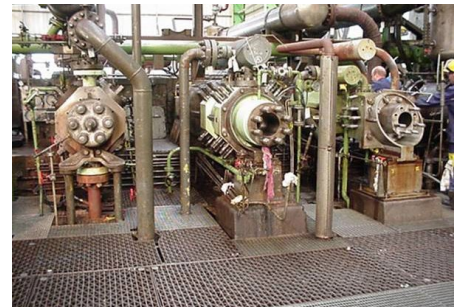
Ammonia plant compressor
