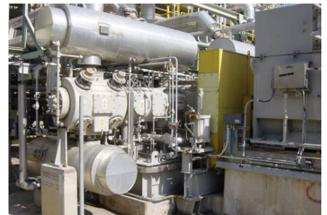
One of the three hydrogen compressors
